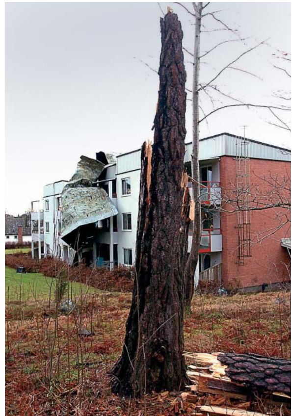
Fig. 15. Storm damage to a residential building in Växjö, southern Sweden (source: Smålandsposten )
